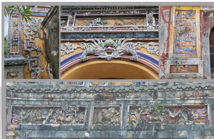
Figure 58 Dragon on the gate to Hue Citadel (Actually taken from July 5 to 7, 2022)
