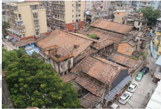
Figure 7 The former residence of Supervisory Censor Sun under restoration. source: Sun Wei, 2021.8.20,Photography
