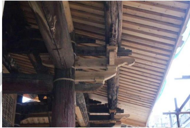
Figure 20: The Ming dynasty's rear gable bucket truss beams in Supervisory Censor Sun's former residence are mostly one, with a square end of rather simple replacement wood, only the edges are sawn into some curves, and the surfaces are not carved.
