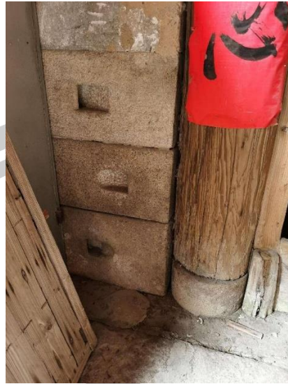
Figure 34 Practicing stones on the wall of the former residence of Supervisory Censor Sun before restoration.
