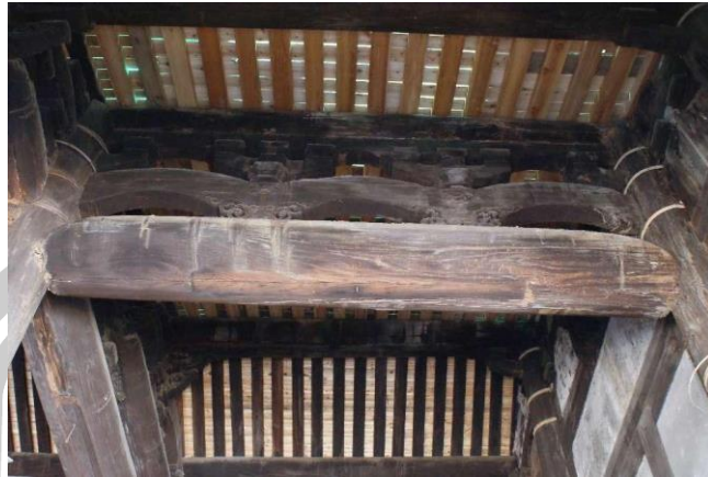
Figure 23 Early wooden structures are characterized by "fat beams and fat pillars", which are also called "melon pillars" and "pork belly pillars" by local people.
