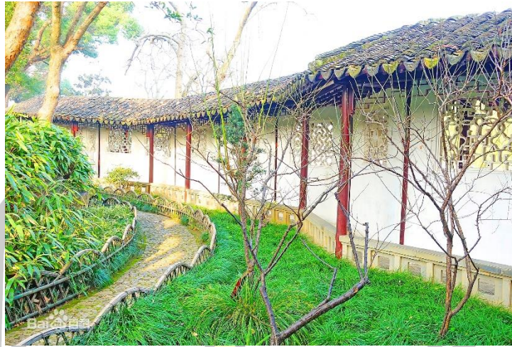
Figure 40 The leaking window of Canglang Pavilion
