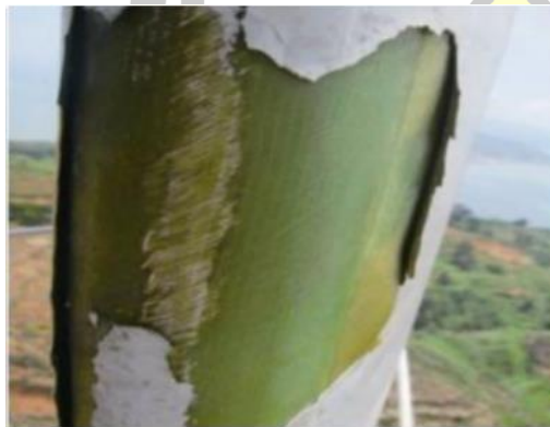
(c) Electrochemical Corrosion
