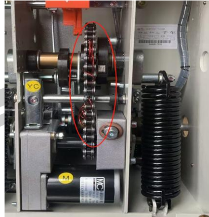
Figure 23 Stuck Energy Storage Mechanism
