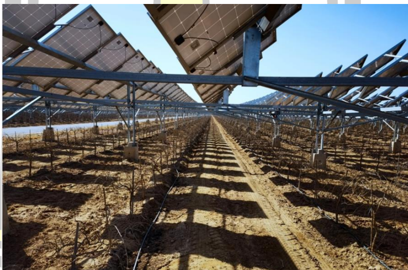
Figure 6 Photovoltaic power station
